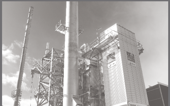
SILVER FERN FARMS BFB BOILER
